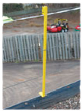
Mid-rail cable supports hold cable a proper height between stanchions.
