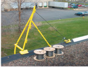
Unused cable remains on spool at end of cable run. No need to cut cable - ever.
